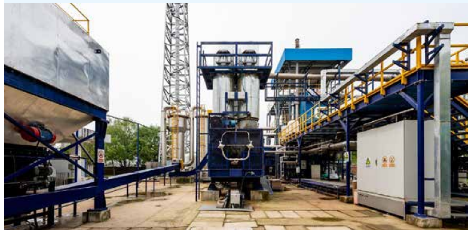
The Omniprocessor, an innovative technology that converts faecal sludge and organic waste into water, energy and other value-added by-products
